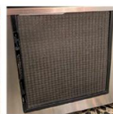
3=Due for cleaning
